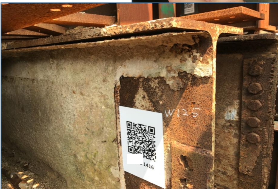
Delamination of steel
